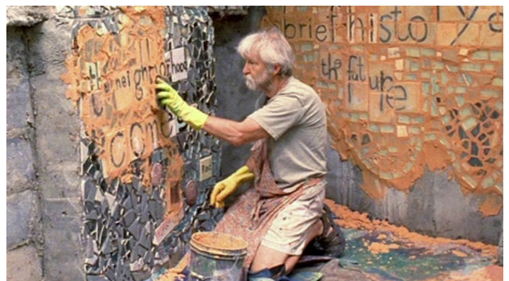
ISAIAH ZAGAR MOSAICKING A WALL IN THE LOWER LEVEL OF PHILADELPHIA'S MAGIC GARDENS
